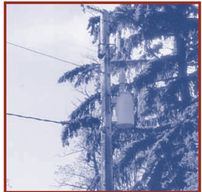
Contact your utility company to clear away vegetation around overhead electrical installations.
